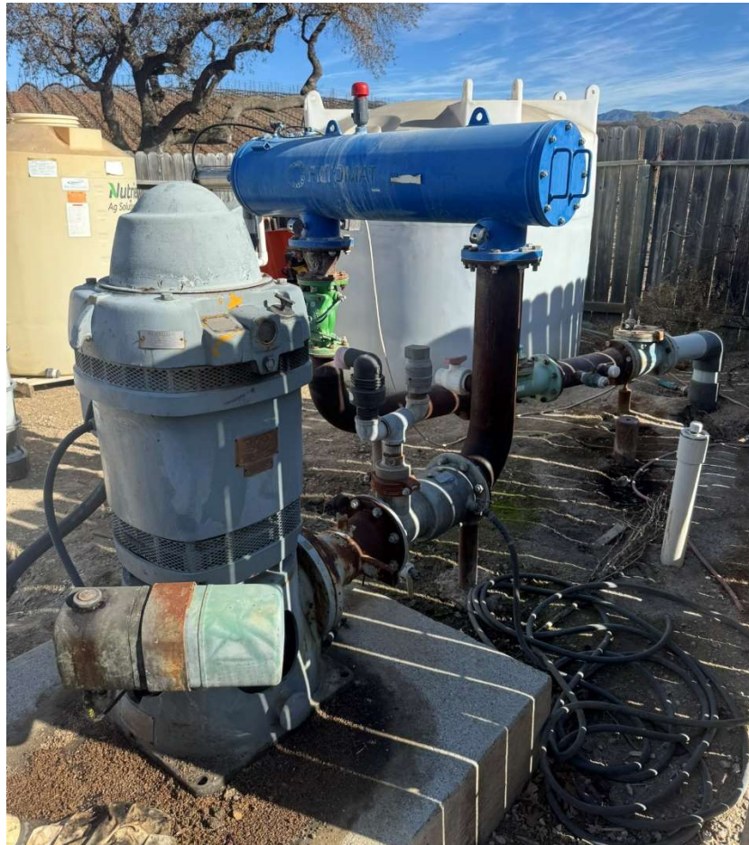
Figure 1a – Vogelzang Vineyard Well Pumping System
