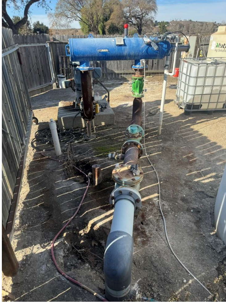
Figure 1b – Vogelzang Vineyard Well Pumping System
